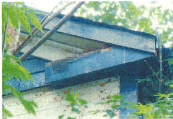
Figure #3: Eaves return Courtesy: Ian McGillivray
