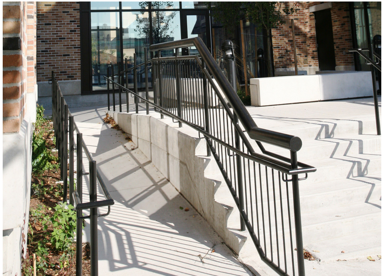
Barrier-free entrances should incorporate ramps, automatic doors, and other elements that contribute to accessibility.
