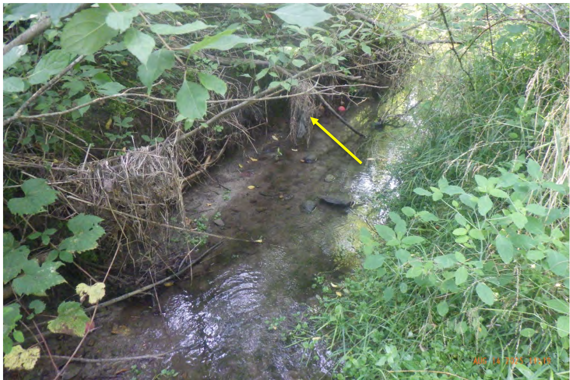
Photo of Reach N-2-D facing downstream. Undercutting was present along the left bank (indicated by arrow).
