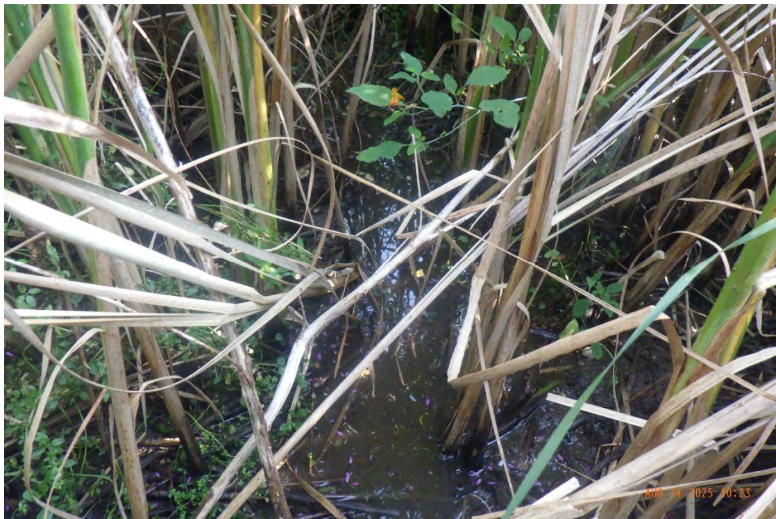
Vegetation was mainly comprised of wetland-type plants that encroached into the low-flow channel. Agricultural fields flanked the reach.
