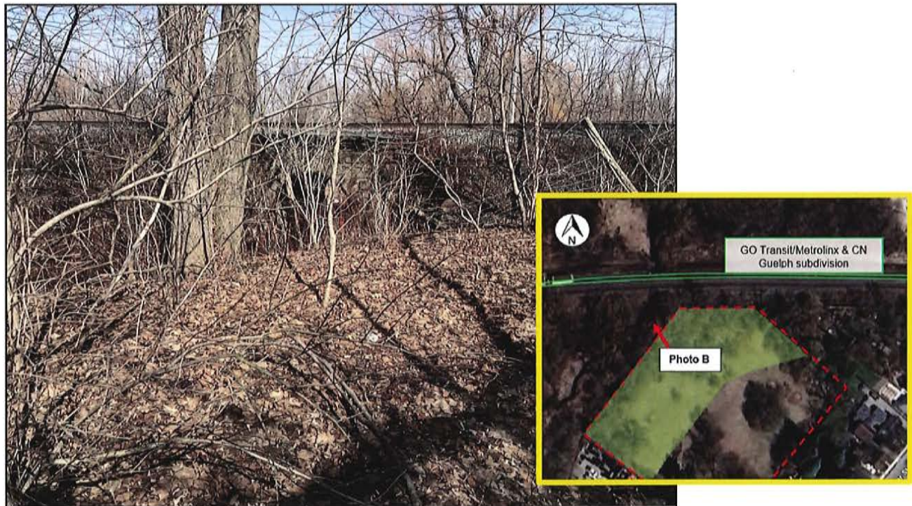
Figure 3: Photo B taken on the site facing the mutual property line showing the existing elevation of the track (top) in relation to the Site (bottom). An existing culvert beneath the railway is part of the watercourse which flows within the environmentally protected lands. Source: Field Photos taken 25-Mar-2026.
